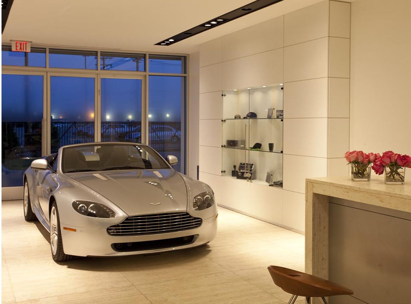
With the 1-x 1-meter travertine panels being pre-fabricated in Italy, it was imperative for installation to be precise. The joints measure 2 mm in width.
